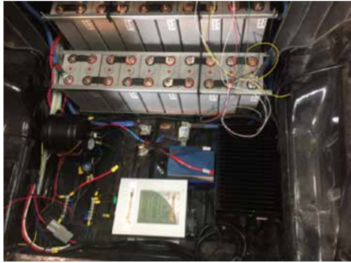
Rear batteries, high voltage charger, DC step down converter to make 12V, aux 12V battery, and air supply for horn. Wiring near completion.
